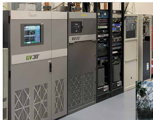
Left: WGCU FM's main transmitter followed by two backup transmitters.
